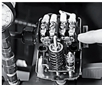
Figure 3 Pressure switch wiring
