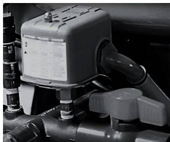
Figure 2 Pressure switch installation
